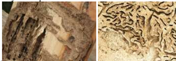
Figure 12: The Termites normal damage (70)
